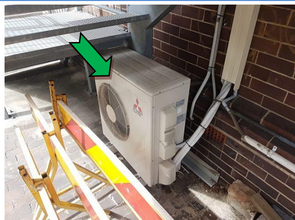
Photo 18. Exterior, ground level, air conditioning unit, unknown refrigerant – suspected non ozone depleting substance.
