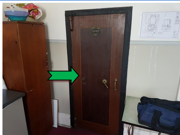
Photo 6. Interior, ground level, community room, strong room – suspected non asbestos-containing door insulation.
