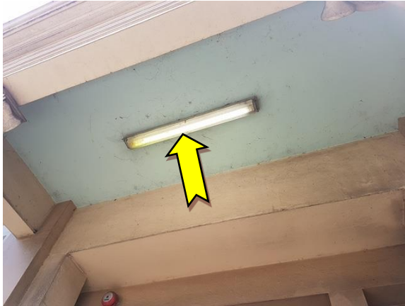
Photo 13. Exterior, entrance, single tube fluorescent light fitting – suspected PCB-containing capacitor.
