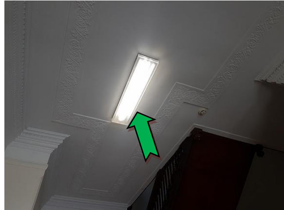
Photo 14. Interior, ground level, throughout, double tube fluorescent light fitting – suspected non PCB-containing capacitor.
