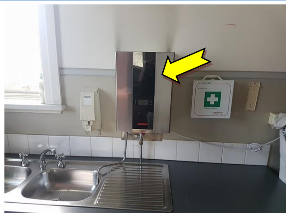
Photo 12. Interior, ground level, community room, kitchenette, hot water heater – suspected SMF internal insulation.
