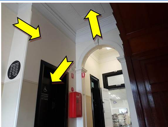
Photo 17. Interior, ground level, throughout, walls, ceiling, doors and door frames – cream, white and black upper coloured paint systems.
