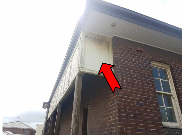
Photo 2. Exterior, west elevation, throughout, high level wall panels – suspected asbestos-containing fibre cement sheeting.
