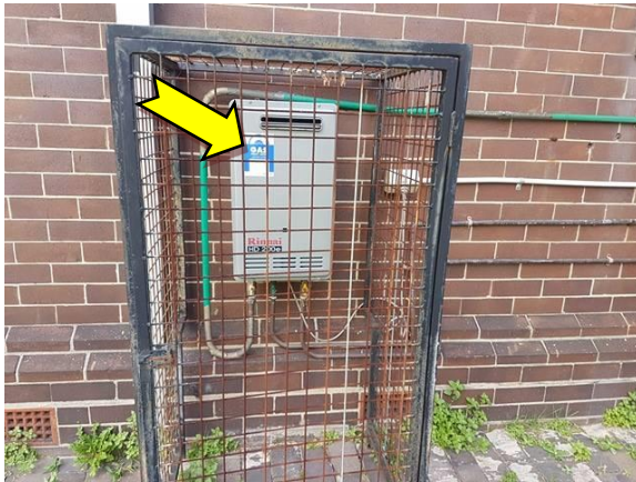
Photo 9. Exterior, south-west elevation, hot water heater – suspected SMF internal insulation.
