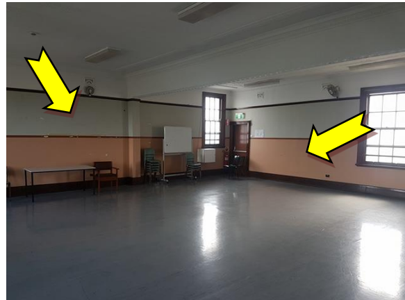
Photo 16. Interior, level 1, throughout, walls – suspected lead-containing cream, and pink upper coloured paint systems.
